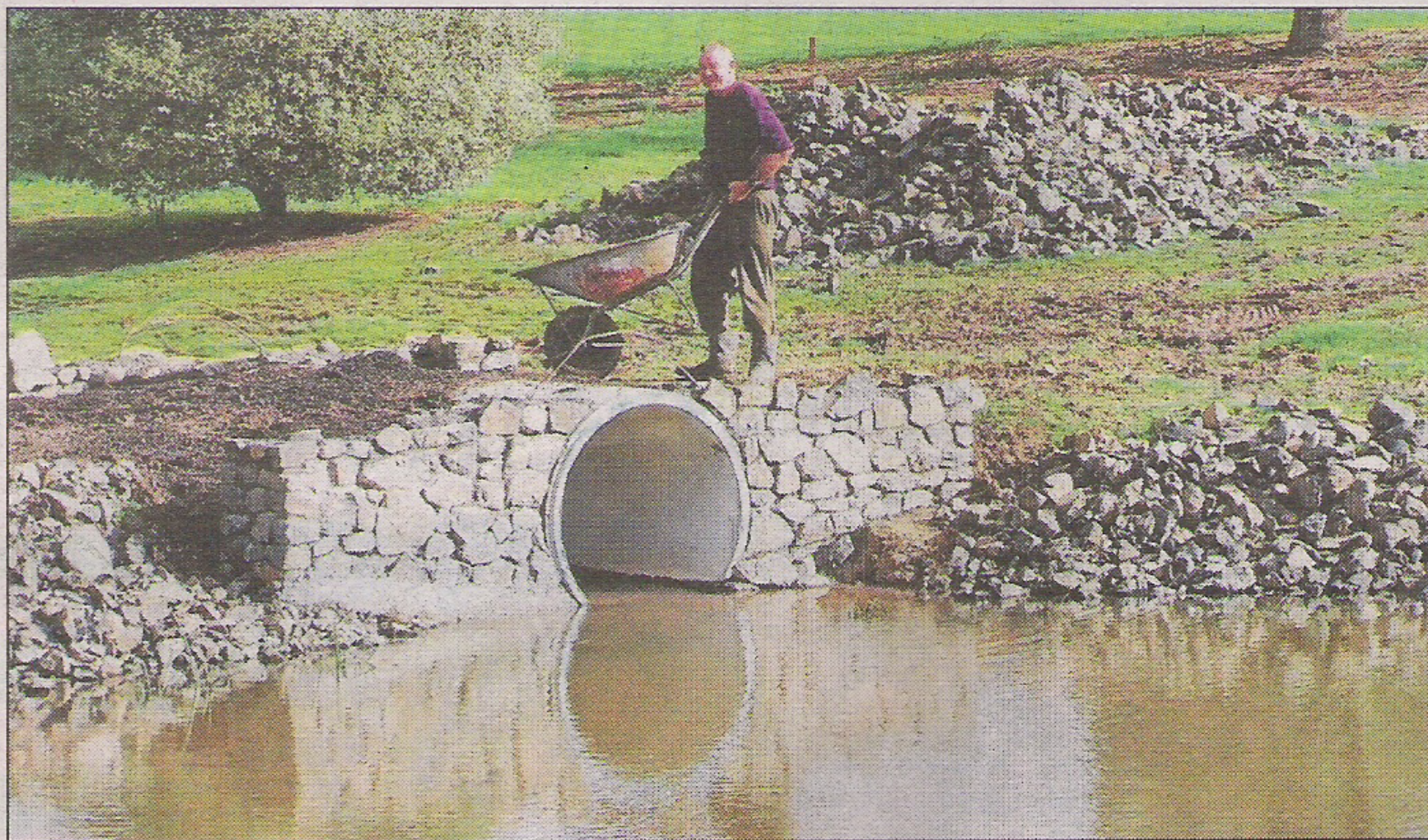
BRIDGE WORK: Rod Price works on the new bridge at the Maramarua Golf Club.
